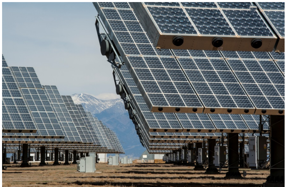
Alamosa Solar Generating Project (Photo credit: Dennis Schroeder, National Renewable Energy Laboratory)
