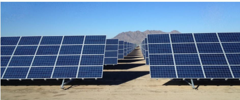
Silver State North Solar Project (Photo credit: R. Sullivan, Argonne National Laboratory)
